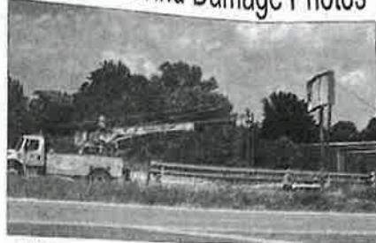
Multiple power poles were snapped on the East side of Highway 49 between SuperValu and McDonalds
