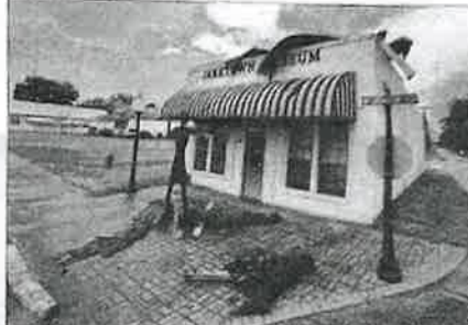
The Jaketown Museum suffered extensive damage to the roof.
