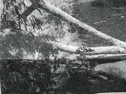
The top of a power pole was snapped off in the alley between Bowles and Mound Streets bringing down utilities.
