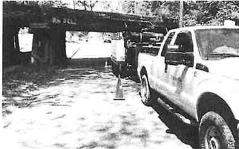
City electric crews were working on Tuesday and will continue working for the rest of the week on South Washington Street changing out utility poles. Please use caution as you travel through this area as traffic may be limited in a single lane. (Photo from Starkville Utilities, for Starkville Daily News)
