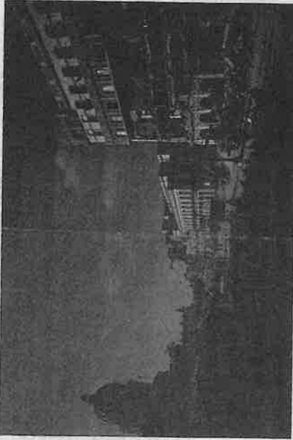
Associated Press | Ramon Espinosa Rescue teams remove debris from the site of a deadly explosion that destroyed the five-star Hotel Saratoga, in Havana, Cuba, Friday.
