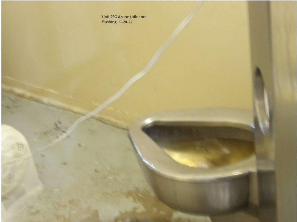
Unit #29 - G-Bldg. toilet will not flush
