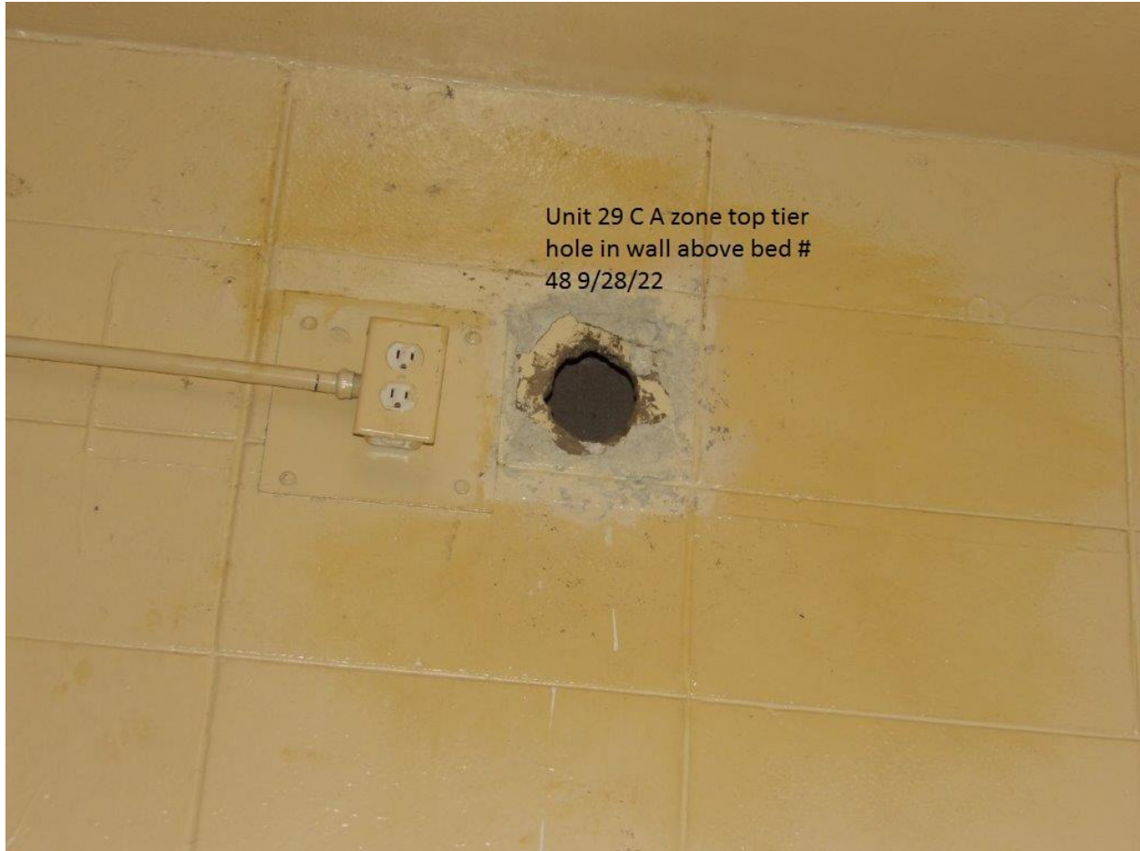
Unit #29 - C-Bldg. A-Zone Top tier has a hole in the wall
