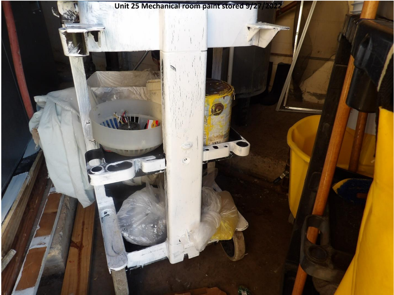
Unit #25 - Mechanical room has paint and chemicals stored in the boiler room
