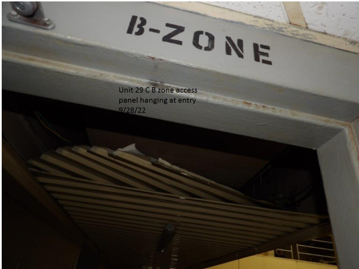
Unit #29 - C-Bldg. B-Zone ceiling metal panel is hanging
