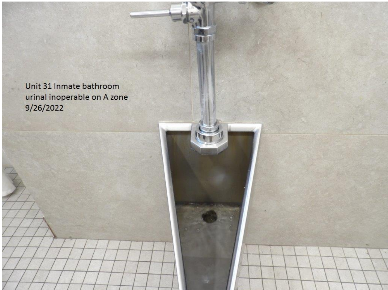
Housing Unit #31 inmate bathroom urinal will not flush
