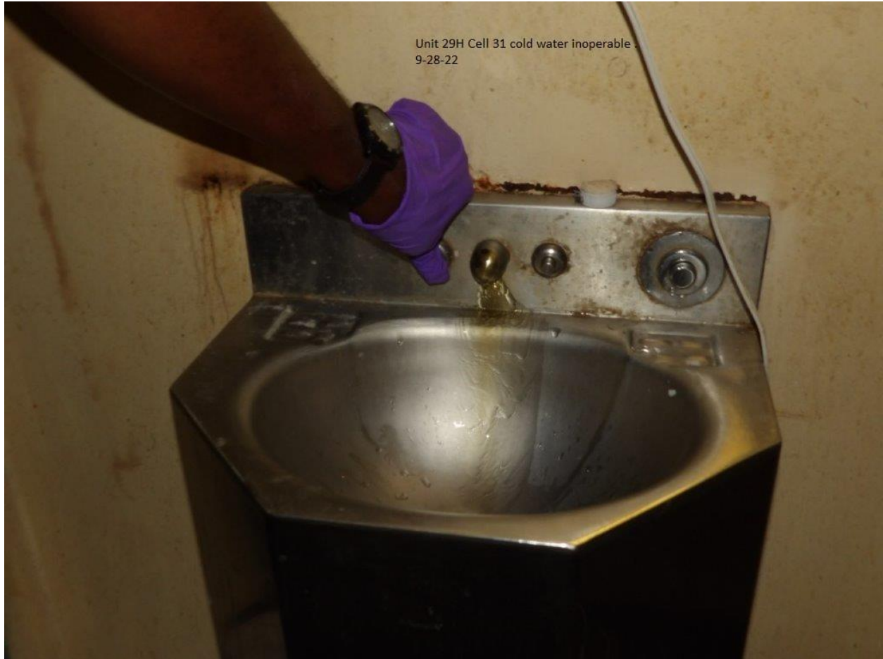
Unit #29 - H-Bldg. A-Zone cell lavatory cold water does not work
