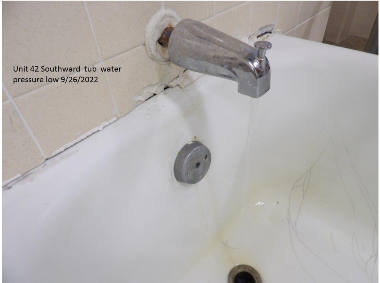
Unit #42 - South wing bathroom water pressure low
