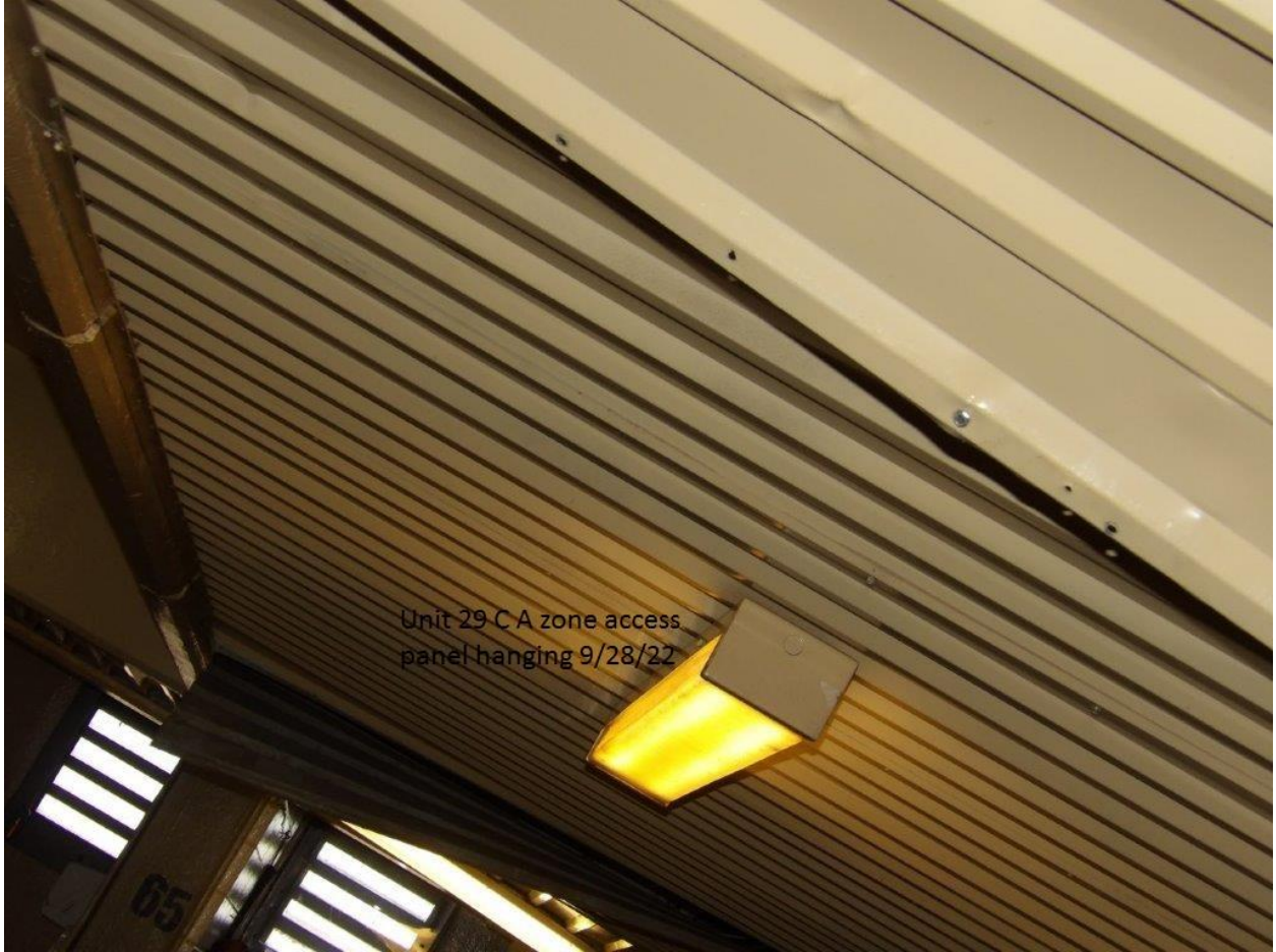
Unit #29 - C-Bldg. A-Zone ceiling metal panel is loose
