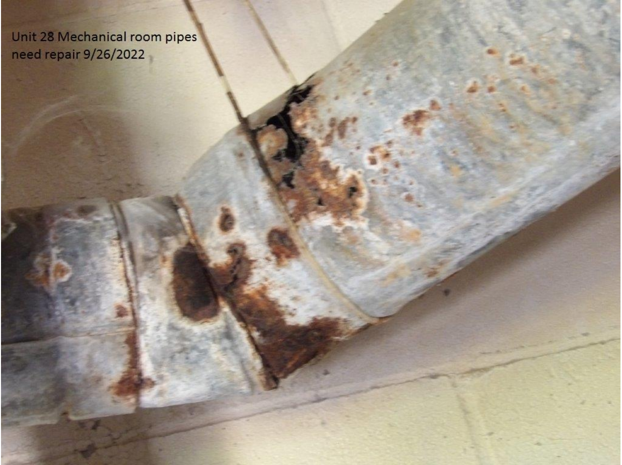
Unit #28 - Mechanical Room boiler has corrosive exhaust pipes
