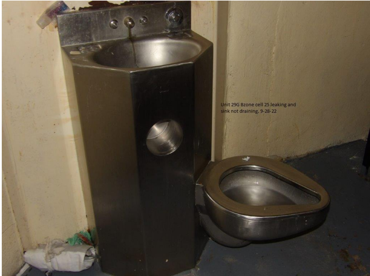
Unit #29 - G-Bldg. B-Zone cell #25 lavatory sink has a leak and is stopped up
