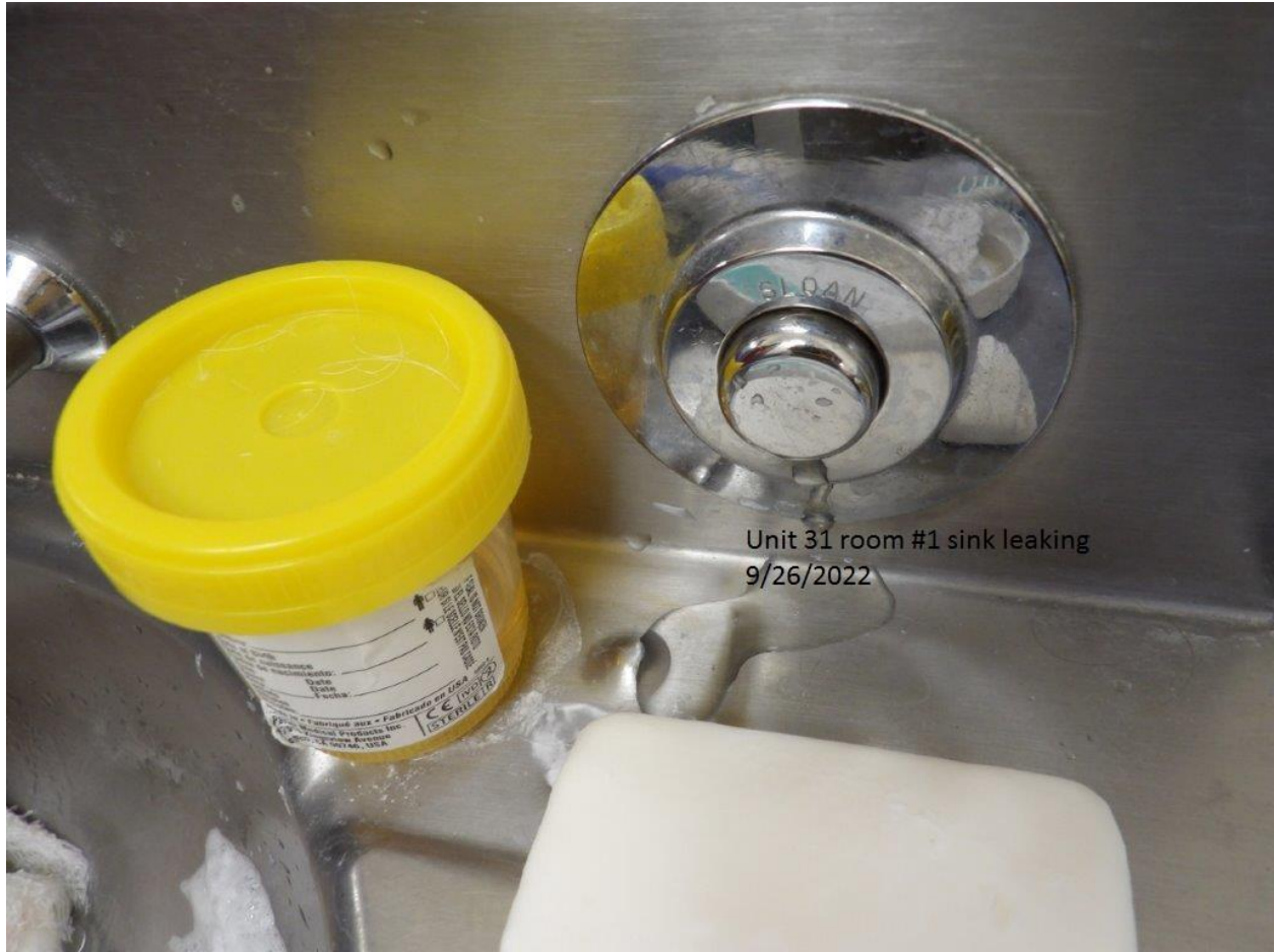
Housing #31 sink leaking
