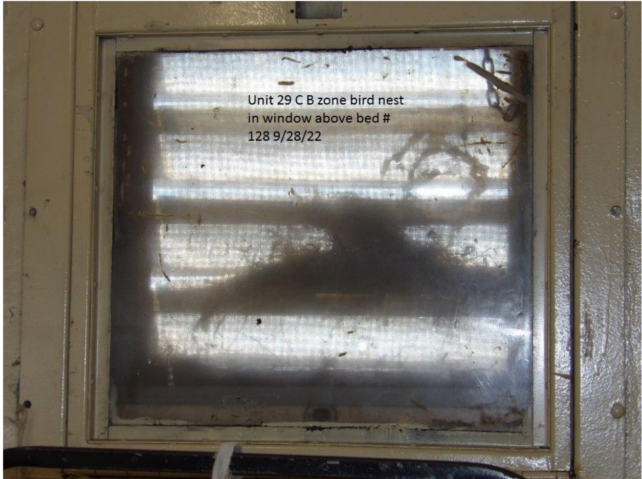
Unit #29 - C-Bldg. B-Zone cell #128 window has a bird nest
