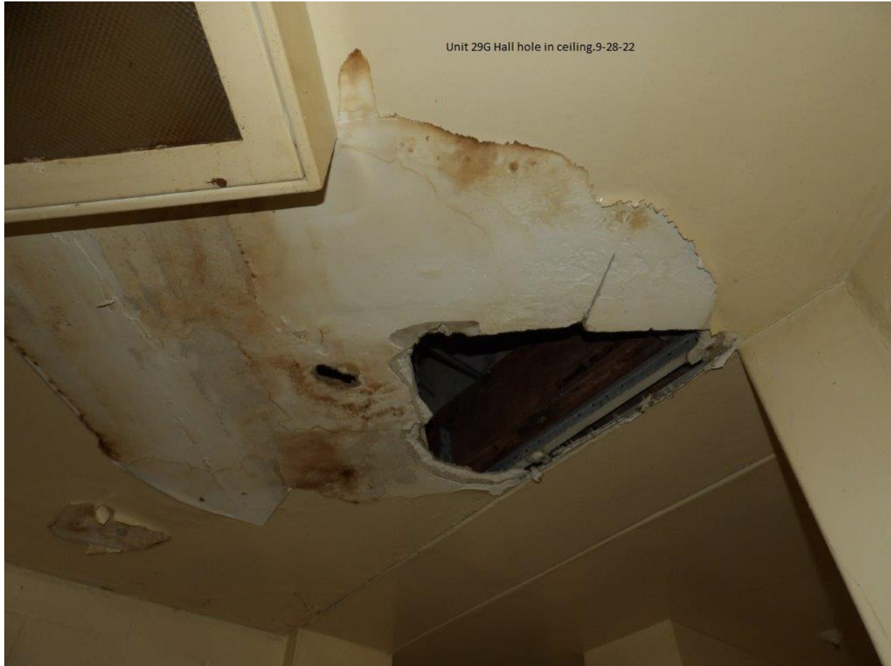
Unit #29 - G-Bldg. hall ceiling has a hole
