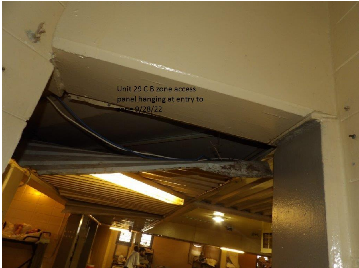
Unit #29 - C-Bldg. A-Zone ceiling metal panel is torn
