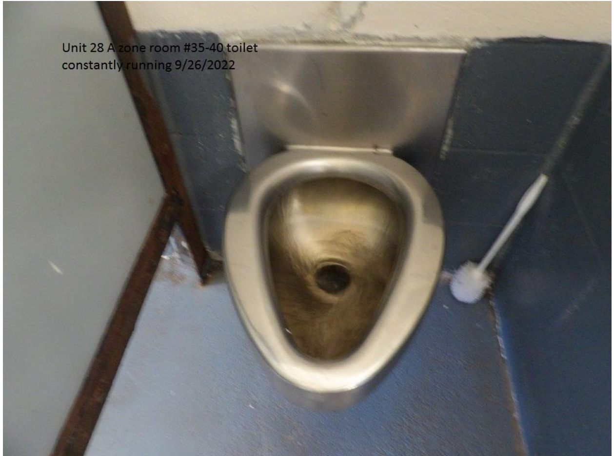
Unit #28 - A-Zone toilet runs water continuously
