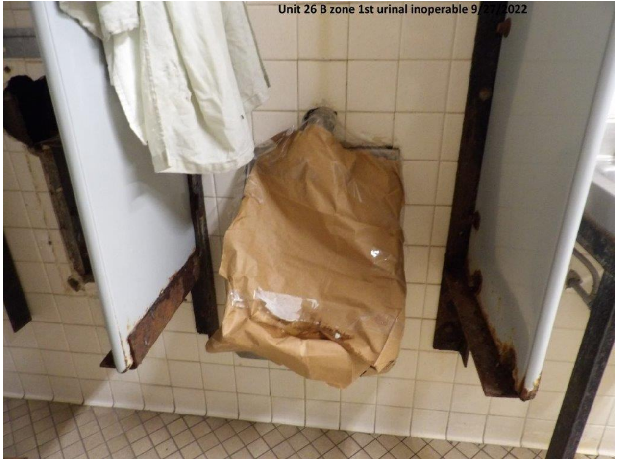
Unit #26 - B-Zone 1 st urinal does not work
