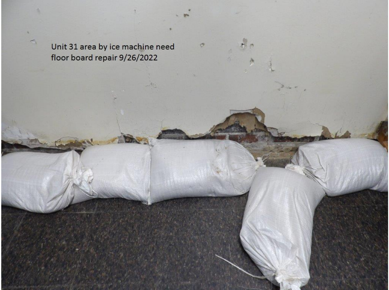
Housing Unit #31 wall near the ice machine damaged by outside flood water
