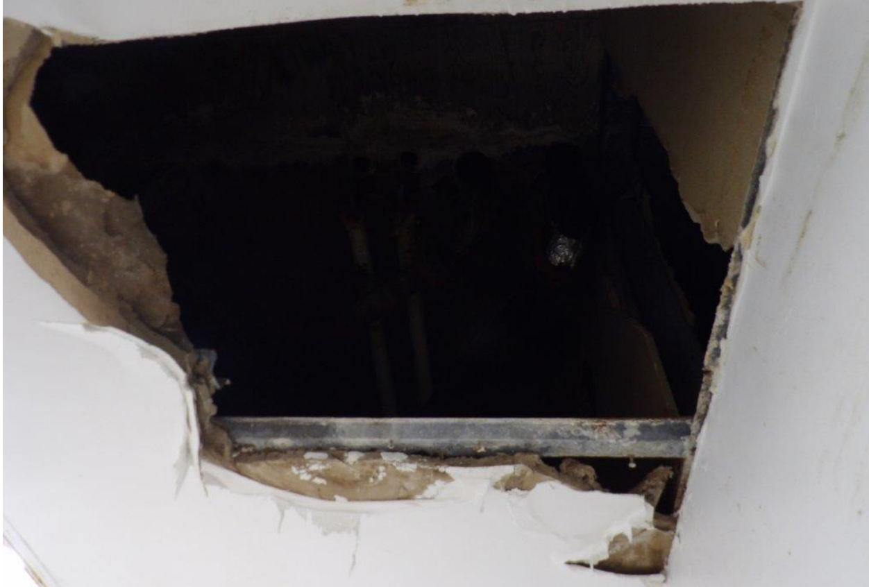
Unit #42 - Laundry Room has hole in the ceiling
