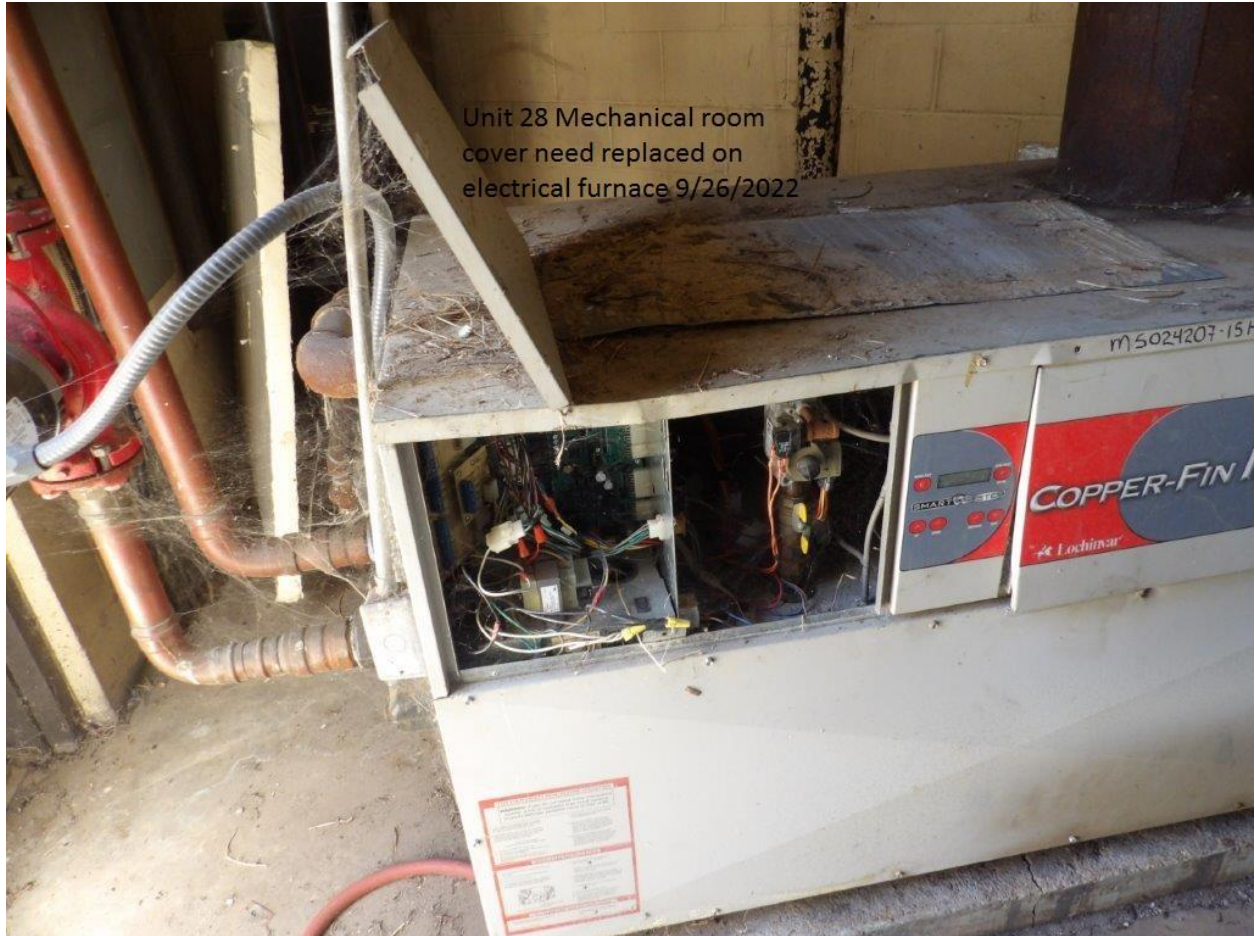
Unit #28 - Mechanical Room furnace door cover missing and has spider webs
