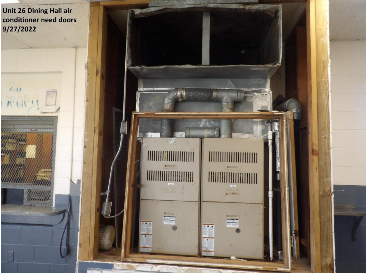
Unit #26 – The kitchen dining hall furnace room doors are missing
