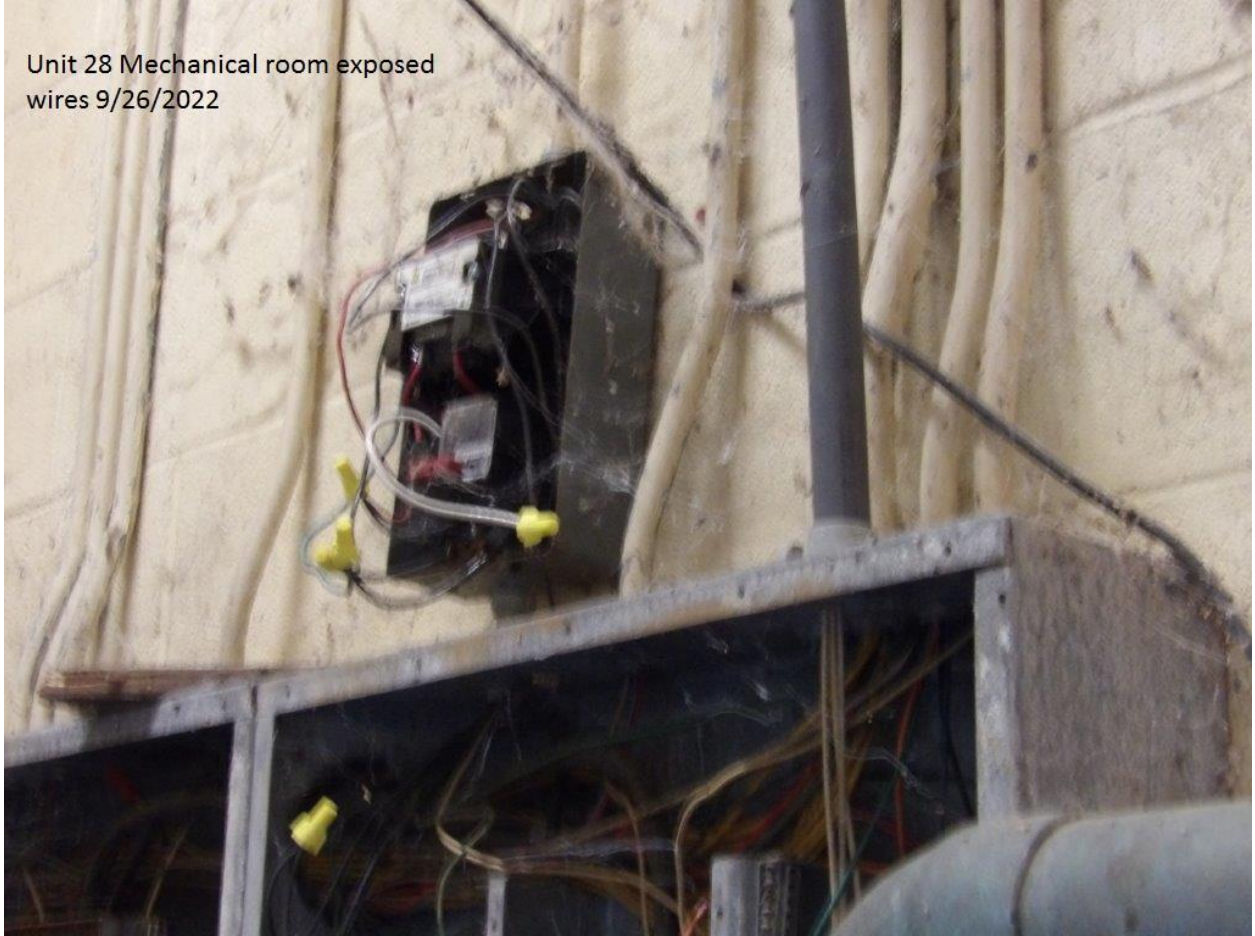
Unit #28 - Mechanical Room has exposed wires
