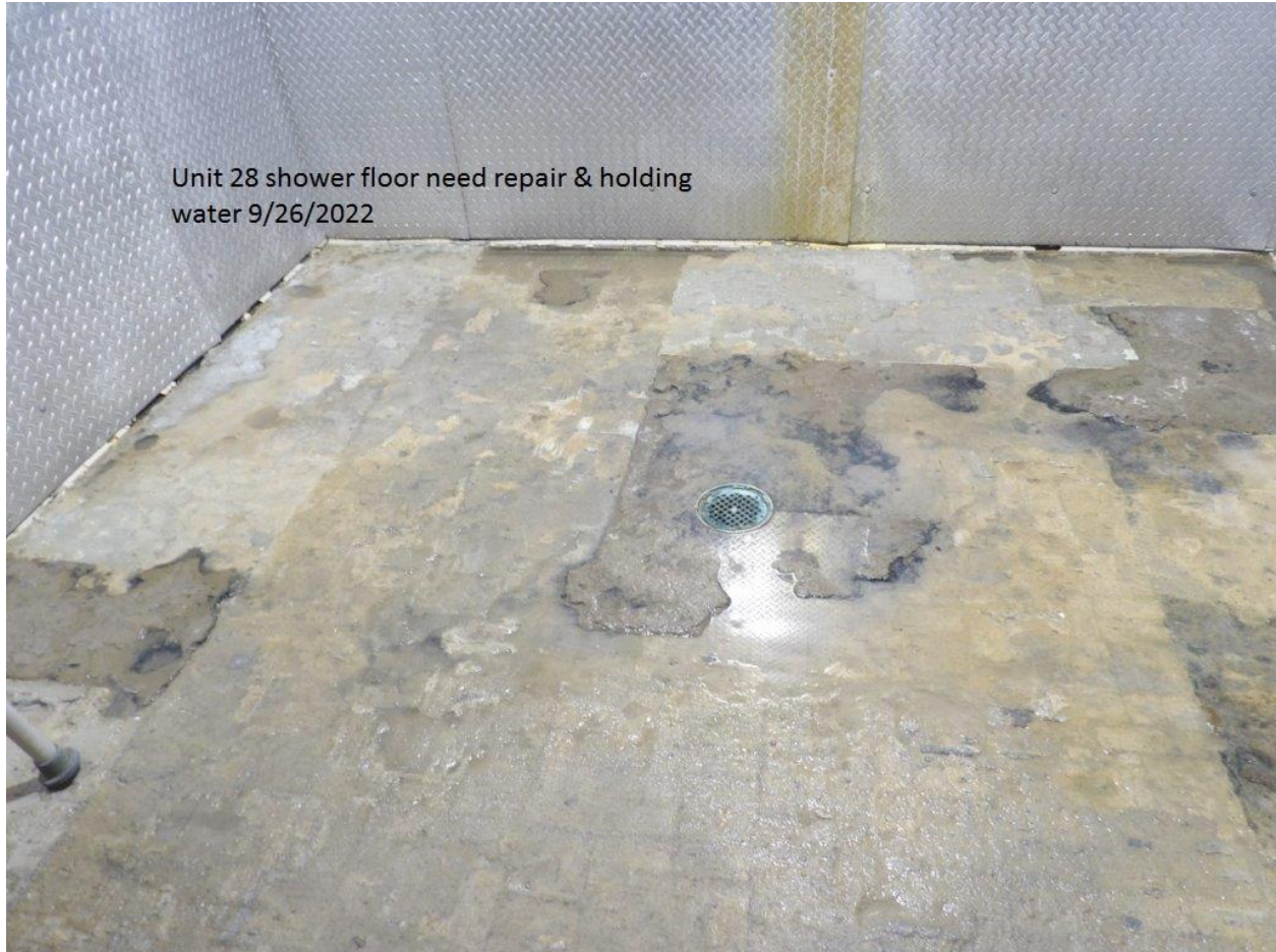
Unit #28 - D-Zone shower is missing tiles and holding water
