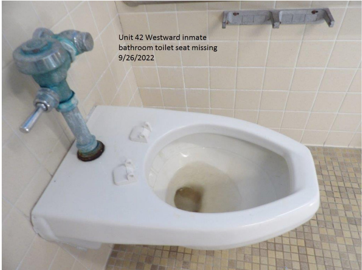
Unit #42 - West wing bathroom toilet seat is missing
