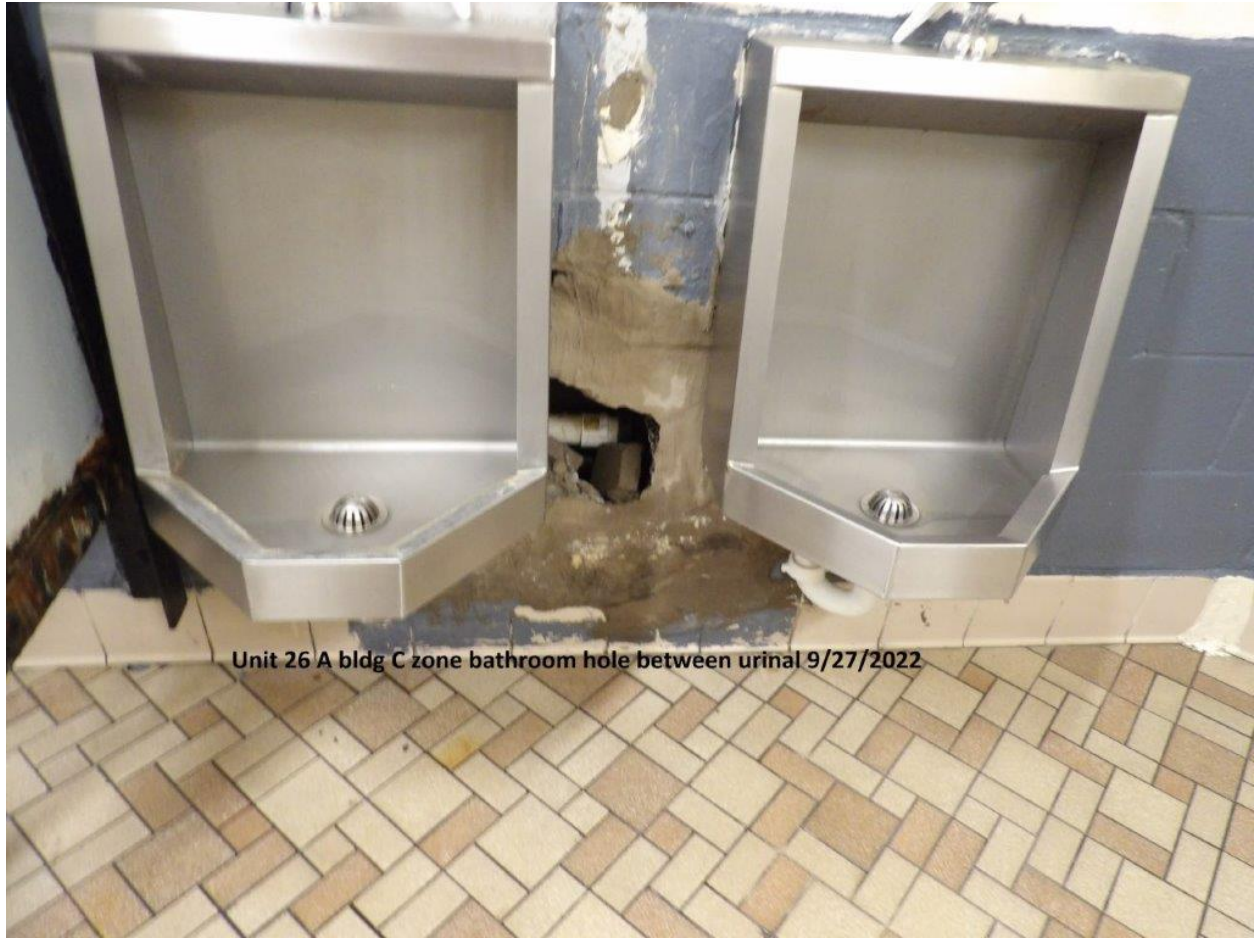
Unit #26 - A-Bldg. C-Zone bathroom wall has a hole between the urinals
