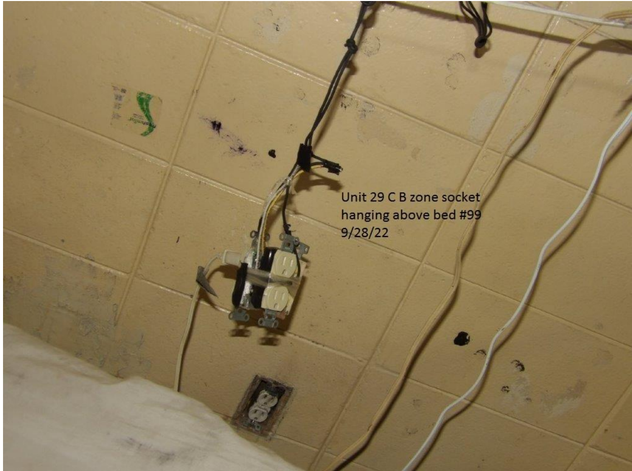
Unit #29 - C-Bldg. B-Zone electrical receptacle is hanging out of the wall
