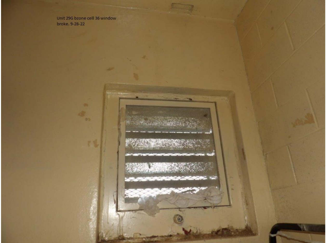
Unit #29 - G-Bldg. B-Zone cell #36 window is broken
