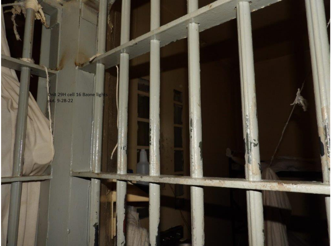
Unit #29 - H-Bldg. B-Zone cell light does not work
