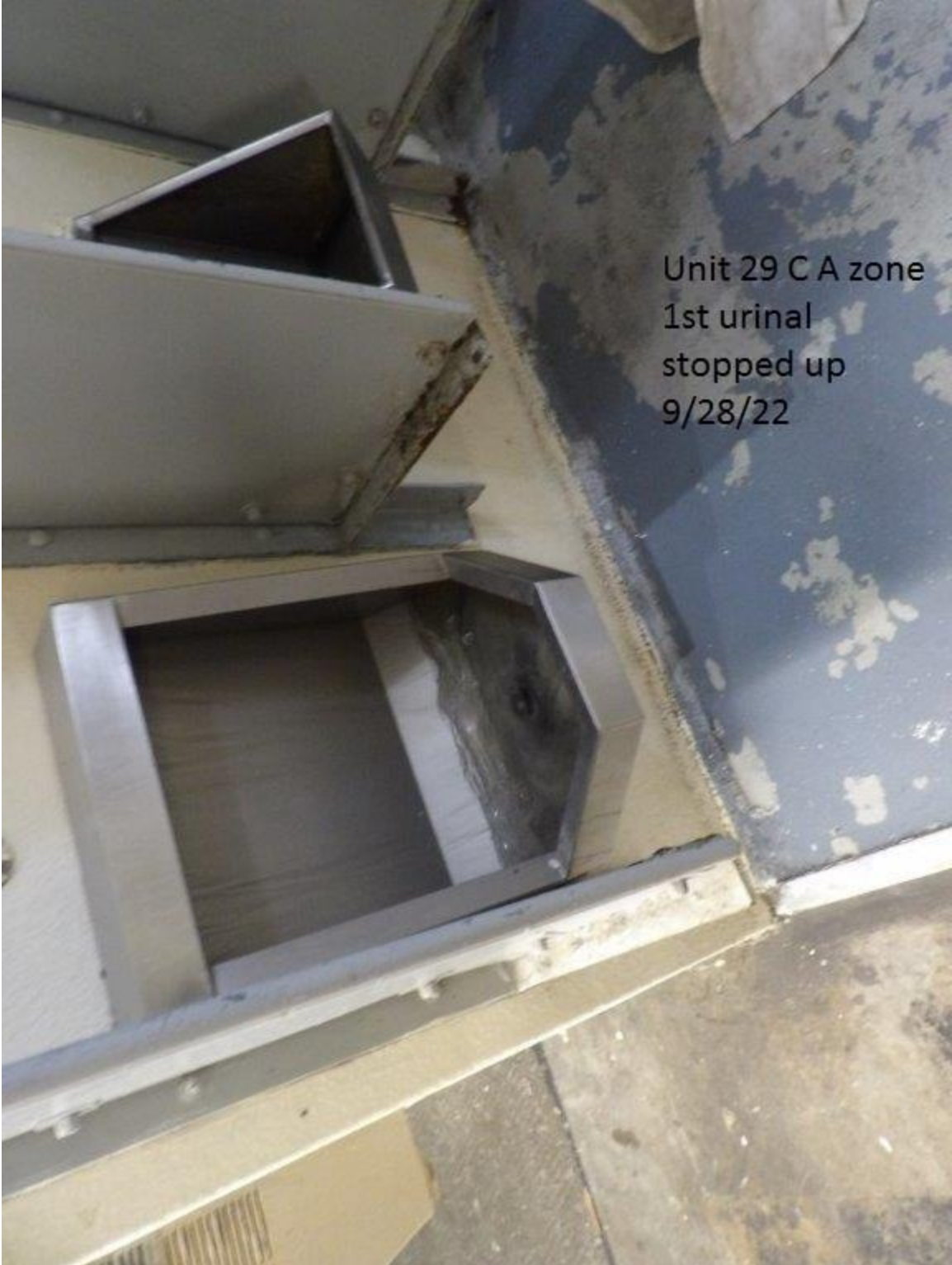
Unit #29 - C-Bldg. A-Zone 1 st urinal is stopped up
