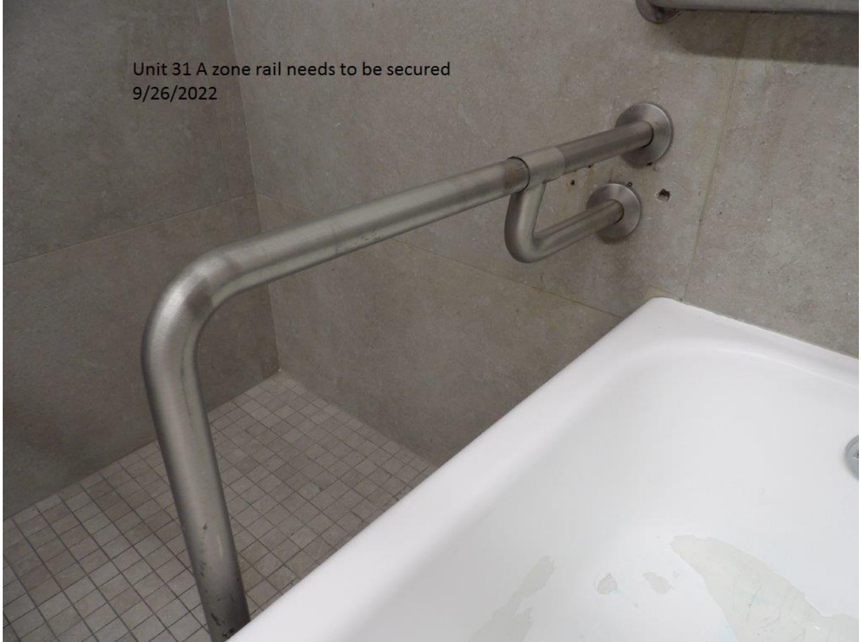
Housing Unit #31 A-Zone handicap handle is loose from the bathtub
