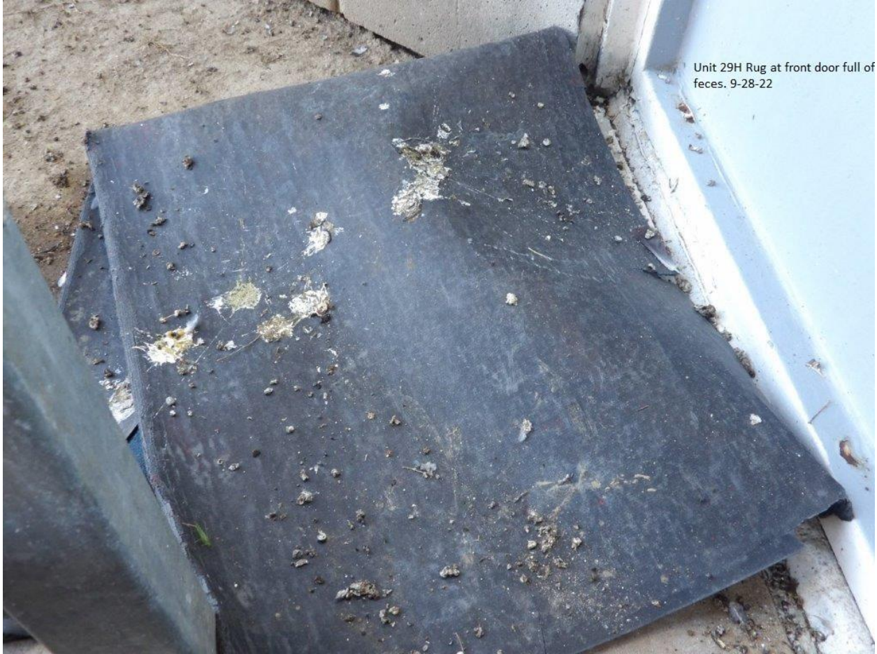
Unit #29 - H-Bldg. The entrance floor mat is covered with bird feces
