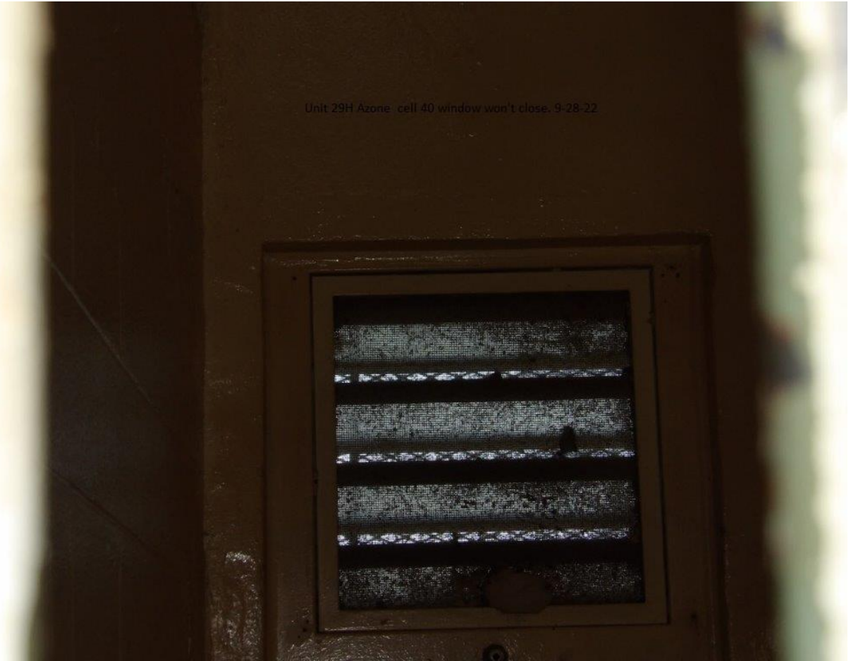
Unit #29 - H-Bldg. A-Zone cell window will not close
