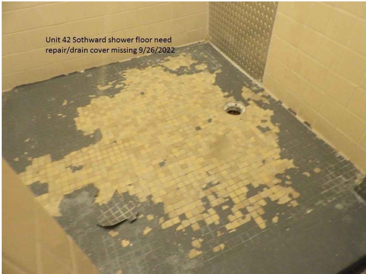
Unit #42 - South wing shower floor has paint peeling and drain cover is missing
