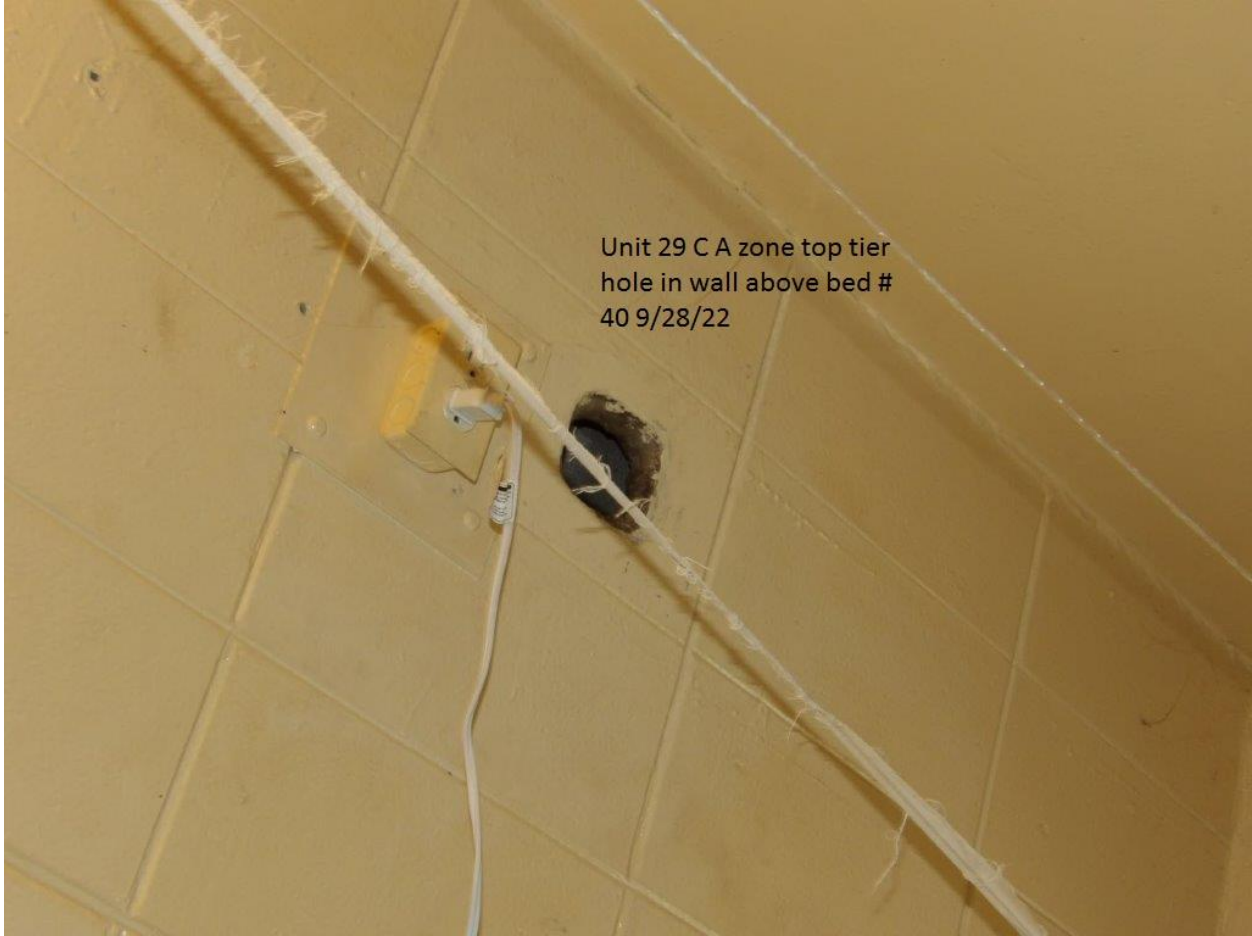
Unit #29 - C-Bldg. A-Zone Top tier has a hole in the wall above bed #40
