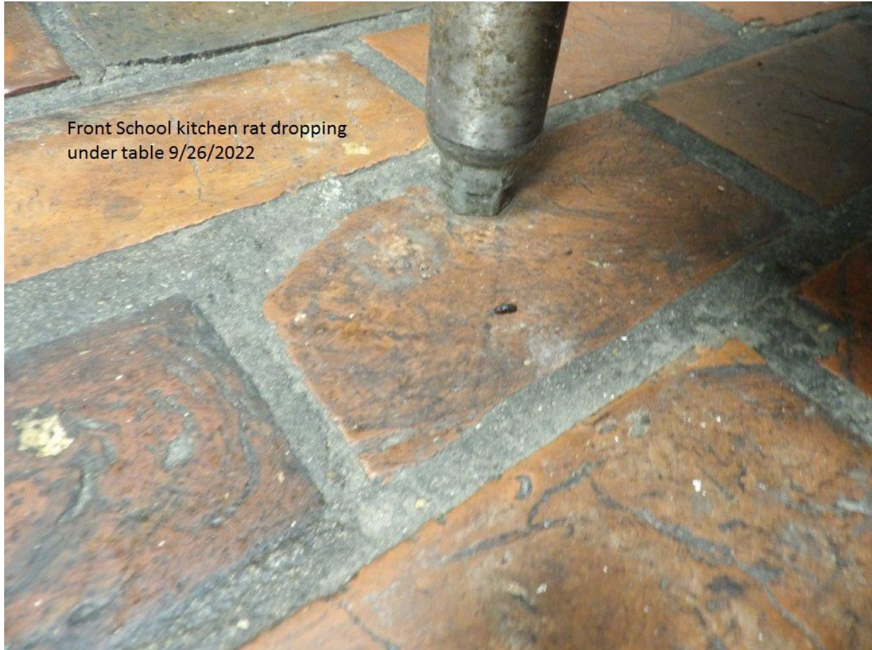
Front School kitchen rat droppings underneath the table on floor
