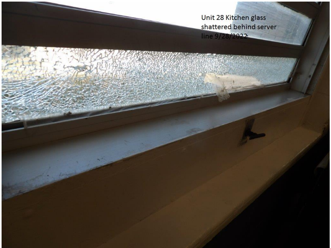
Unit #28 Kitchen window shattered
