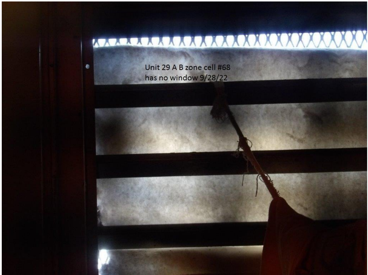
Unit #29 - A-Bldg. B-Zone cell #68 window is missing and light does not work
